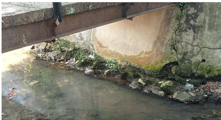
DINDING PENAHAN TANAH RETAK
