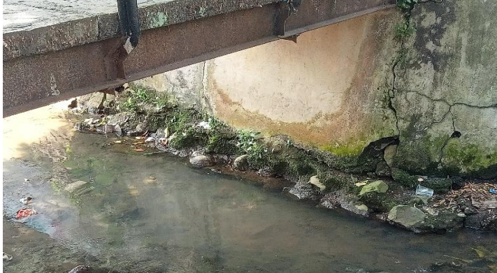
DINDING PENAHAN TANAH RETAK
