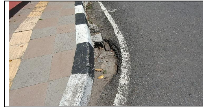
PIPA CUCURAN DRAINASE TERSUMBAT
