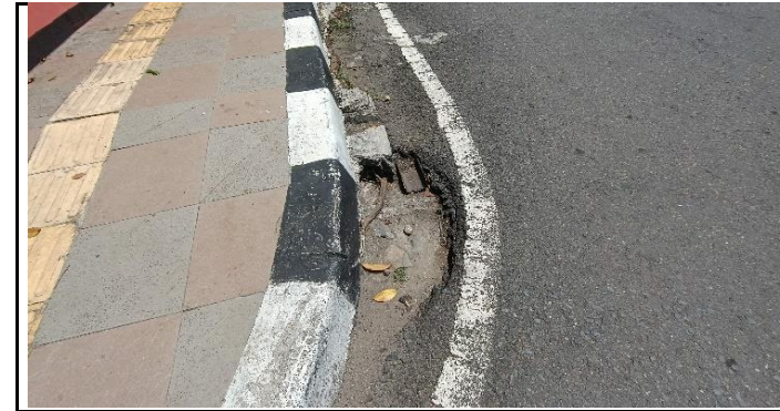
PIPA CUCURAN DRAINASE TERSUMBAT
