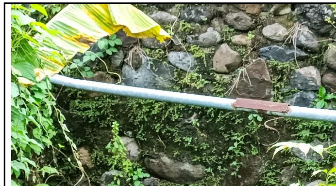
PIPA UTILITAS AIR MINUM
