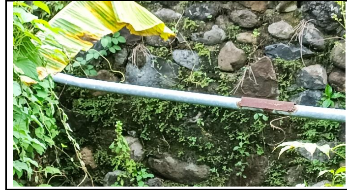
PIPA UTILITAS AIR MINUM
