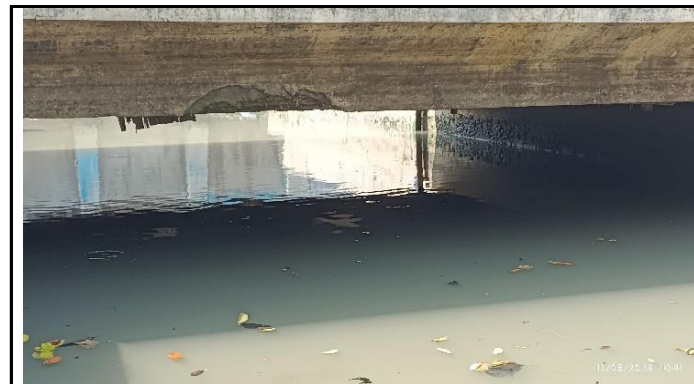
GELAGAR BETON KEROPOS
