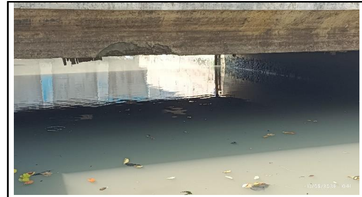
GELAGAR BETON KEROPOS
