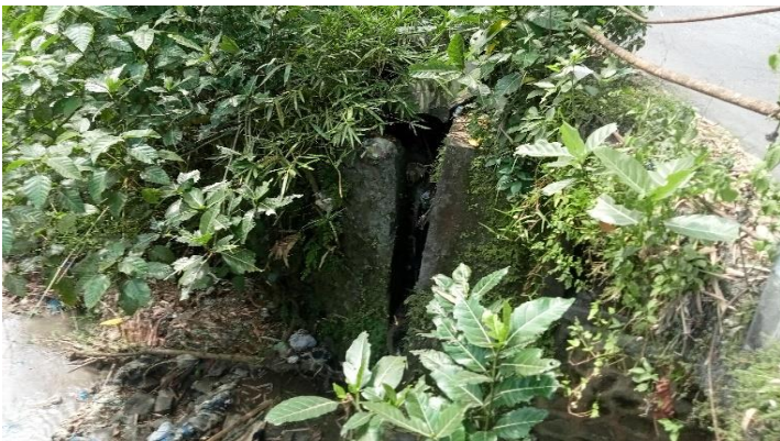
DINDING PENAHAN TANAH PECAH
