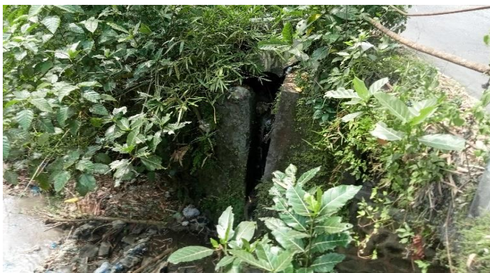
DINDING PENAHAN TANAH PECAH
