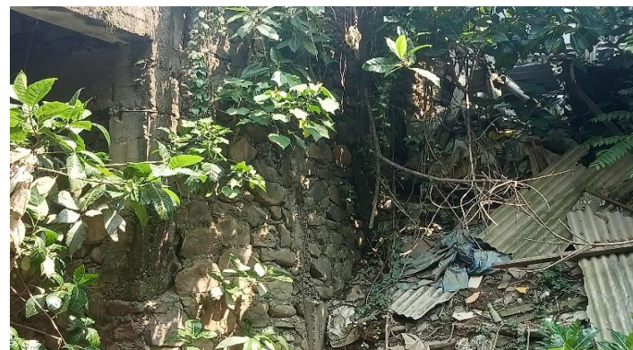
DINDING PENAHAN TANAH PECAH
