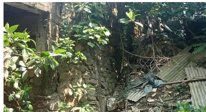
DINDING PENAHAN TANAH PECAH
