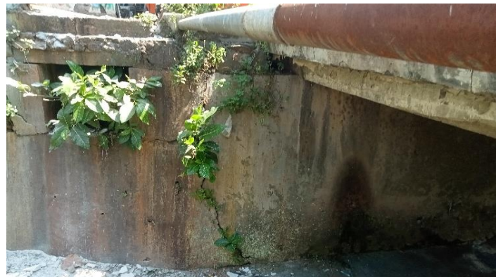
DINDING PENAHAN TANAH PECAH
