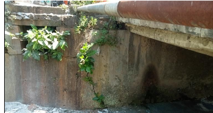
DINDING PENAHAN TANAH PECAH
