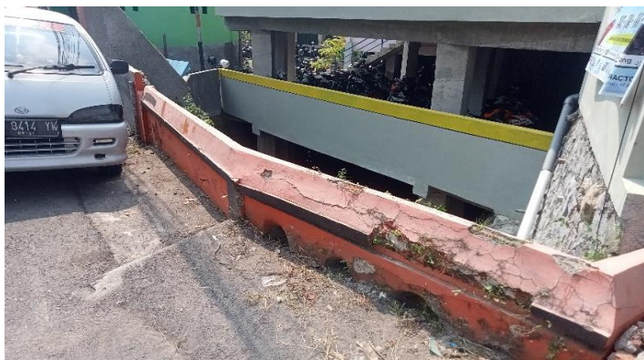
SANDARAN / PARAPET PECAH
