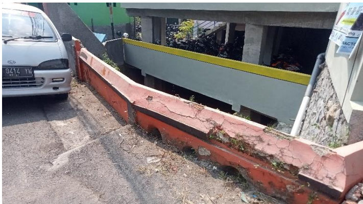
SANDARAN / PARAPET PECAH
