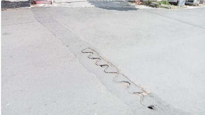
EXPANSIONT JOINT MENGLUPAS
