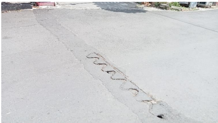
EXPANSIONT JOINT MENGLUPAS
