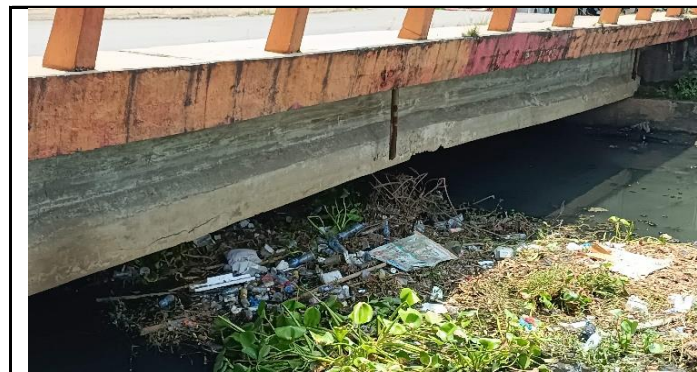
GELAGAR BETON KEROPOS
