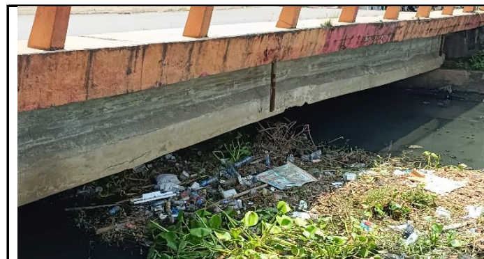
GELAGAR BETON KEROPOS
