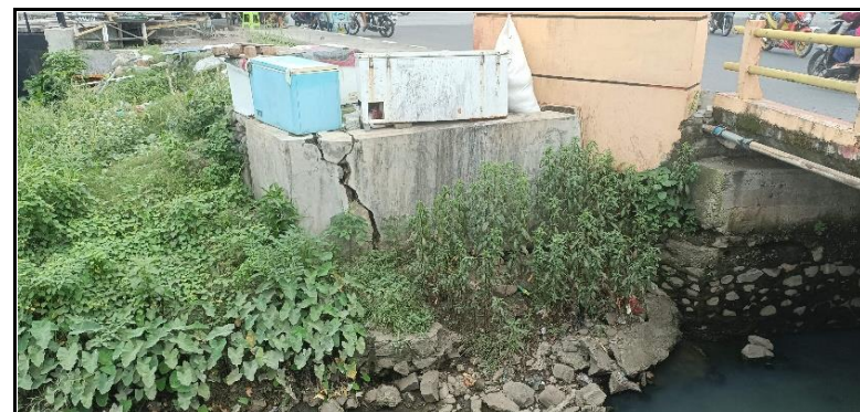
DINDING PENAHAN TANAH (TEMBOK SAYAP) RETAK
