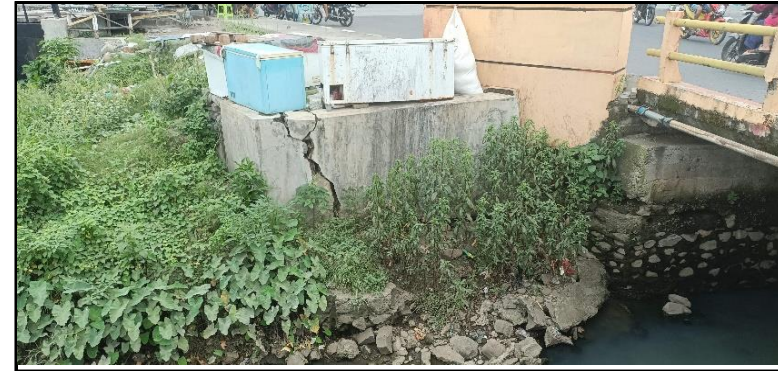
DINDING PENAHAN TANAH (TEMBOK SAYAP) RETAK
