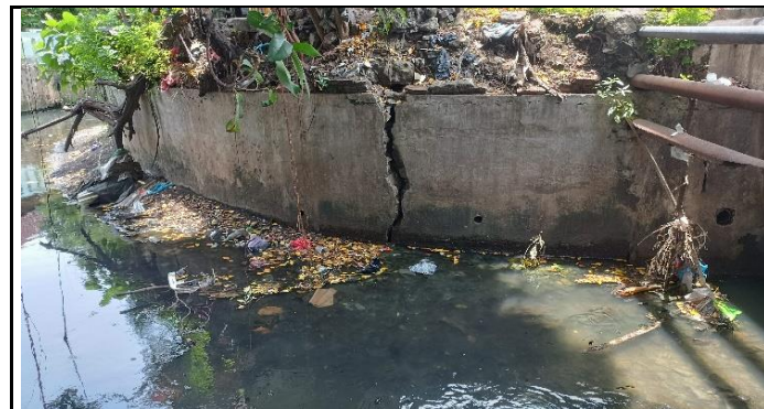
DINDING PENAHAN TANAH RETAK
