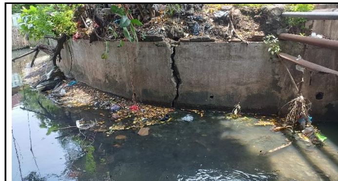
DINDING PENAHAN TANAH RETAK
