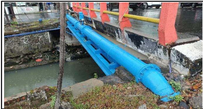
UTILITAS PIPA AIR MINUM
