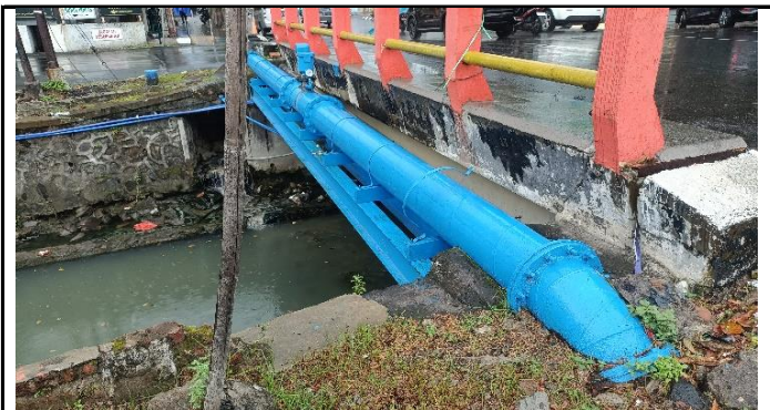
UTILITAS PIPA AIR MINUM
